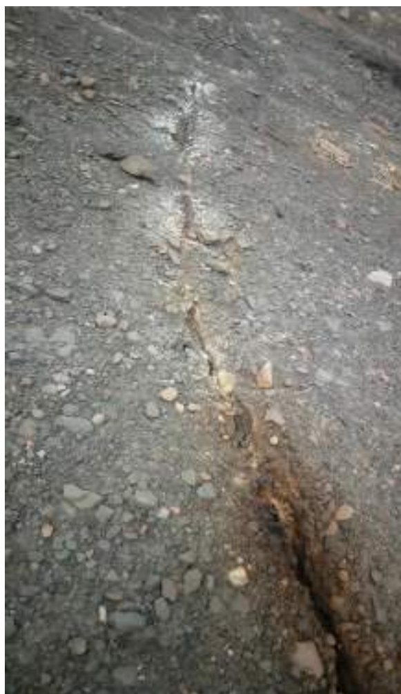
Figure 20: Fume cracks in the Bhulanbarari area.
